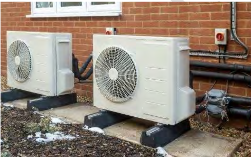
Figure 7: An Air Source Heat Pump
